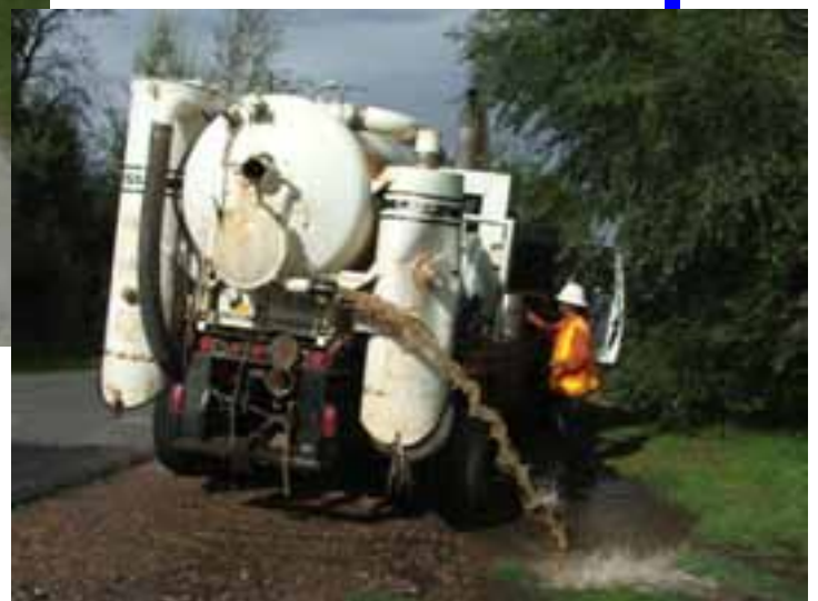
Drilling fluid being dumped into a roadside ditch.
